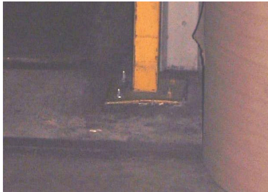
Figure 13. Raised guard rail brackets caused a significant contact risk to raw material stock
